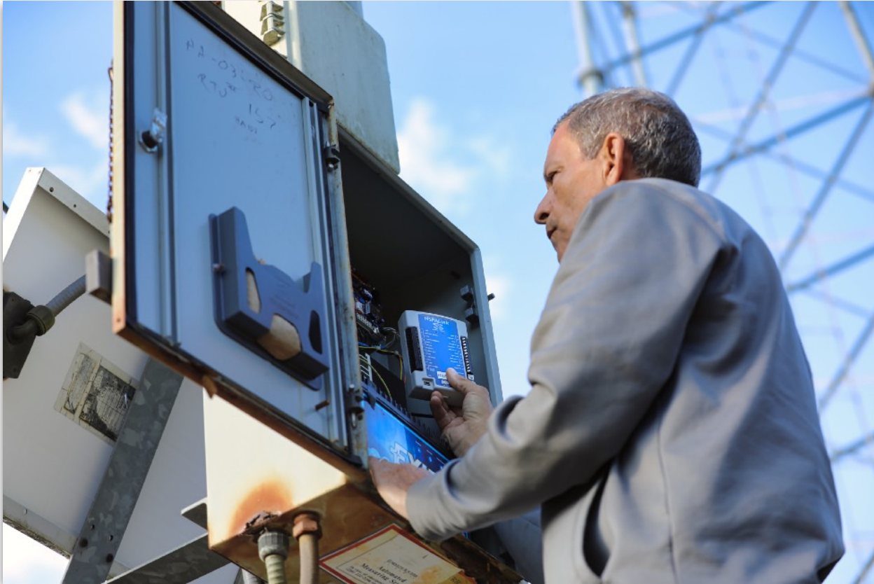
EAA's Ron Gloy retrofits a weather station in San Marcos with a new data collector.
